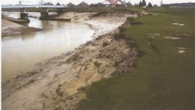
Slumping bank - site of emergency works
