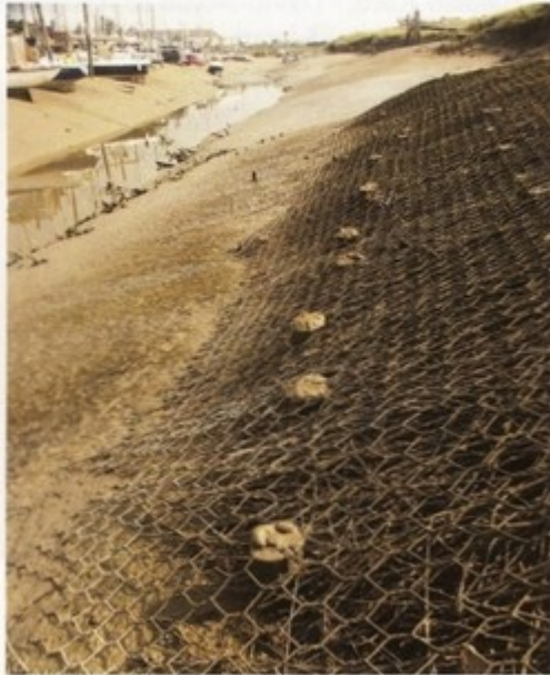
Sedimentation at trial site
