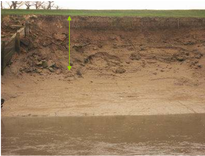
Photograph 3: Scour hole, with 2m vertical face
