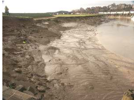
Photo 2: Scour hole at low tide
