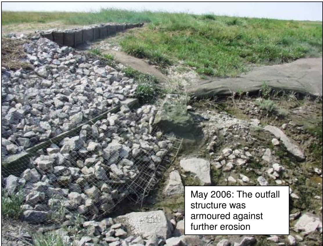
May 2006: Coir logs were installed above the gully to halt flood erosion
